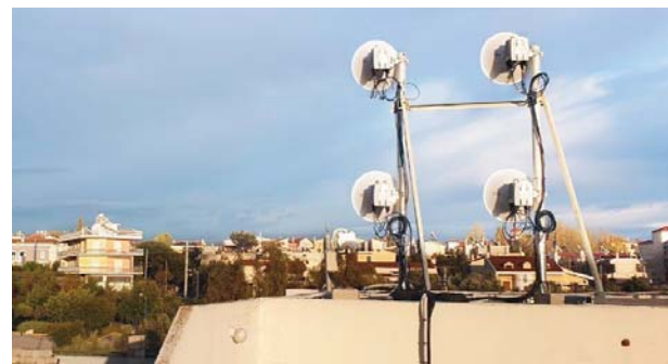
Figure 16. A 100Gbps hop at OTE Academy in Athens, Greece, stretching over 1.5km towards OTE headquarters
